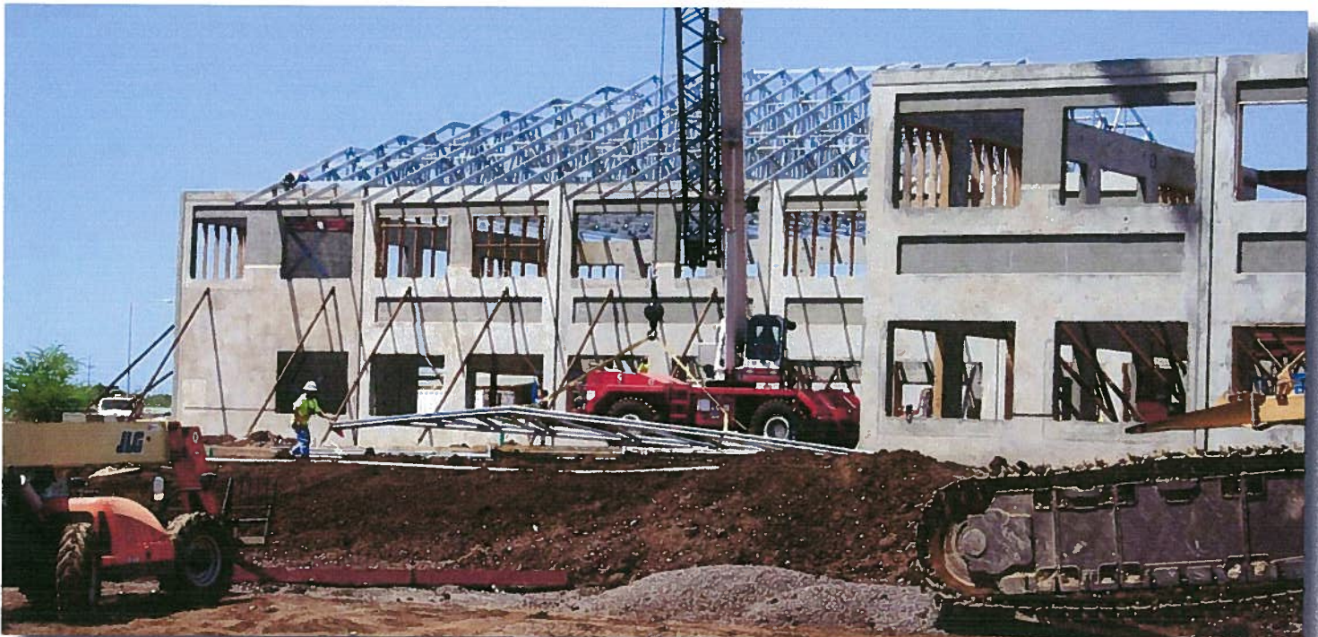
Construction on the Hale Kalaniana‘ole office complex, DHHL’s future home, began in January 2007.
